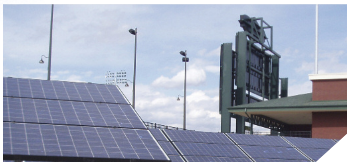
At Dow Diamond, 168 solar panels power the scoreboard and other areas of the stadium.
